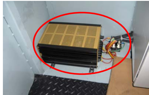
Magnet Power Supply and Relay 69 Detail
